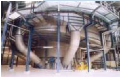
Boilers, Heat Recovery Steam Generators, Air Quality Control Systems
